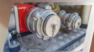
Fire Fighting System
